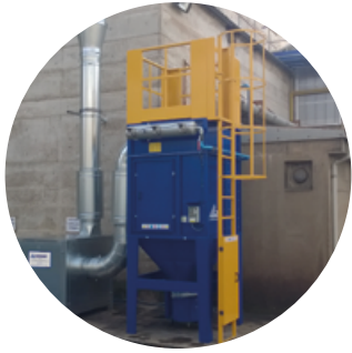
General ventilation and filtration plants
